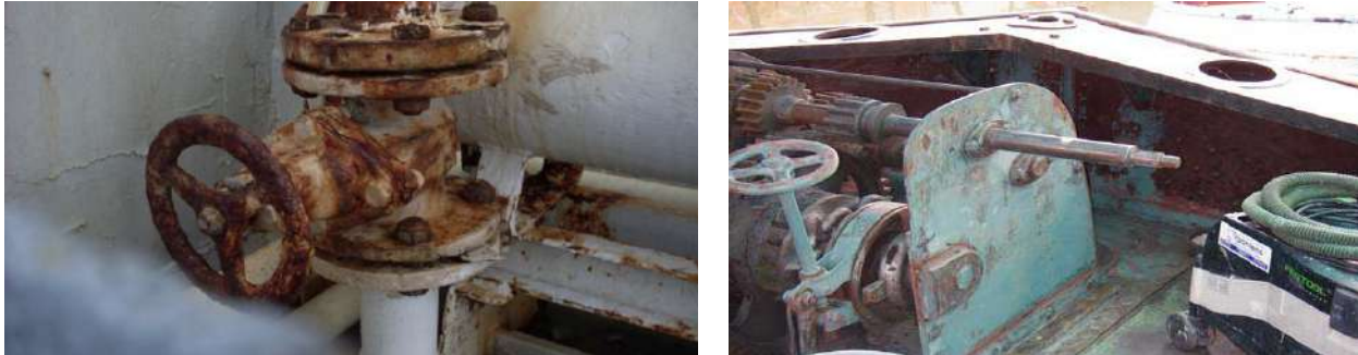
Examples of surfaces unsuitable for repainting
